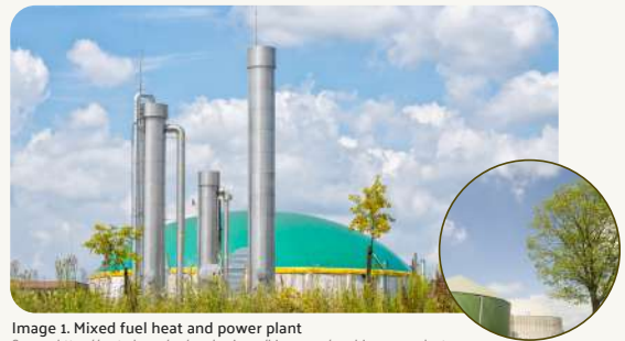
Image 1. Mixed fuel heat and power plant Source: https://orsted.com/en/our-business/bioenergy/our-bioenergy-plants
